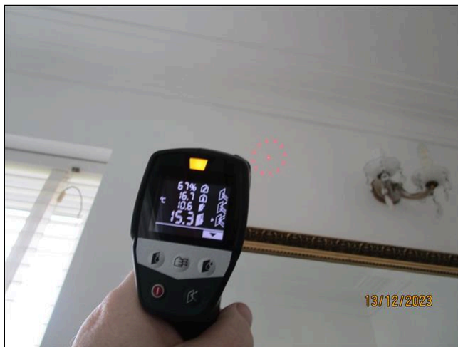
11.0 Item 1(Picture) Raised condensation readings in Bathroom
