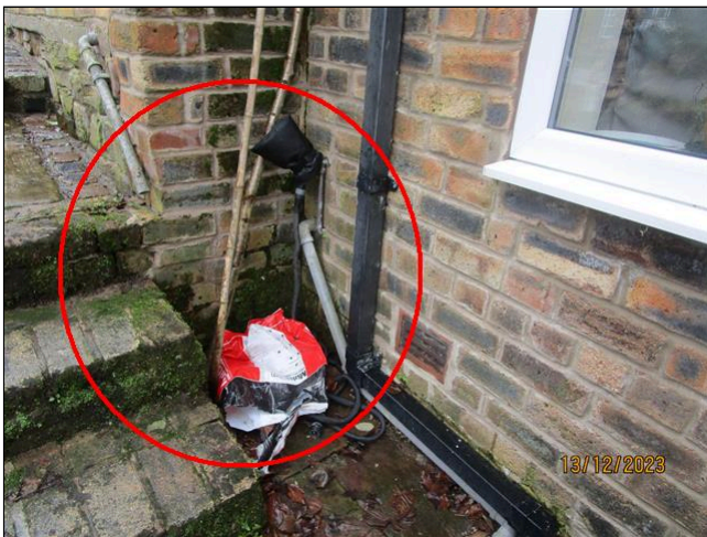
3.0 Item 3(Picture) Raised step and leaking water tap
