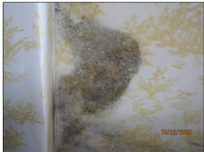
9.2 Item 2(Picture) Black mould on some walls
