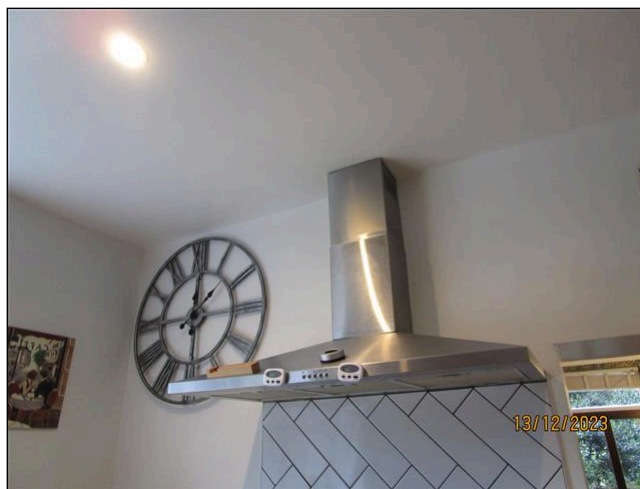
11.1 Item 2(Picture) Vent in Kitchen
