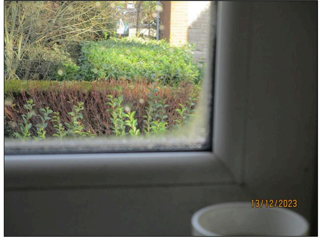
8.2 Item 2(Picture) Water droplets from condensation
