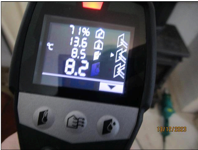
3.2 Item 3(Picture) Condensation occurring in some rooms
