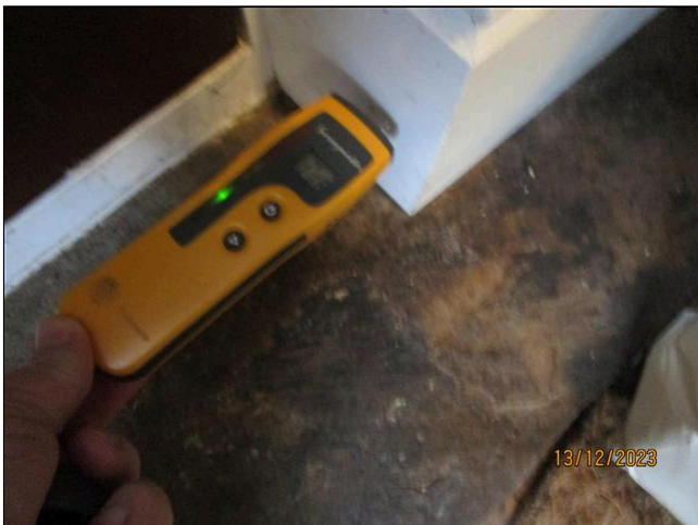
3.0 Item 5(Picture) Damp checks to skirting boards
