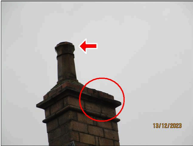
3.0 Item 1(Picture) Chimney no cowl and no vents
