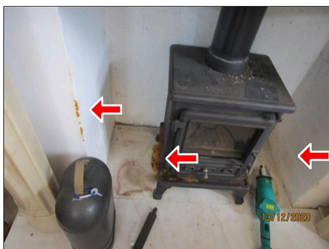
10.2 Item 3(Picture) Rust and damp noted
