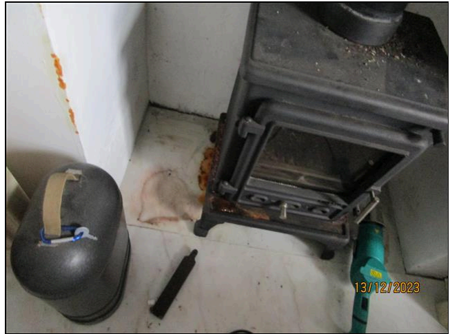
3.0 Item 8(Picture) Damp to chimney breasts
