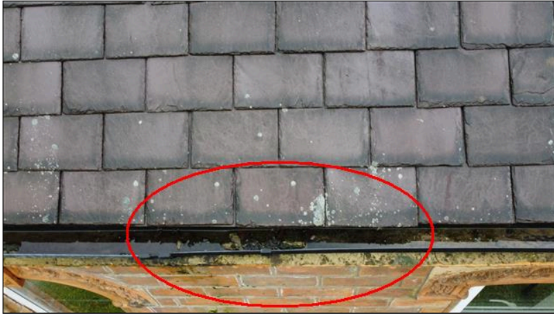
6.2 Item 1(Picture) Gutter leak and standing water
