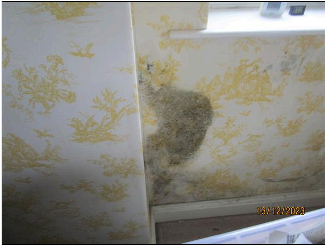
3.0 Item 7(Picture) Black mould in places
