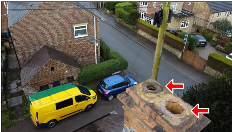
4.2 Item 2(Picture) Holes where pots removed
