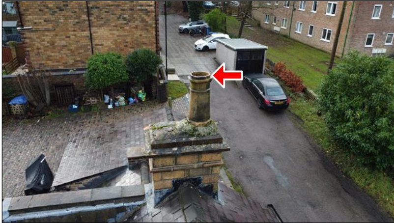
4.2 Item 1(Picture) Chimney no cowl
