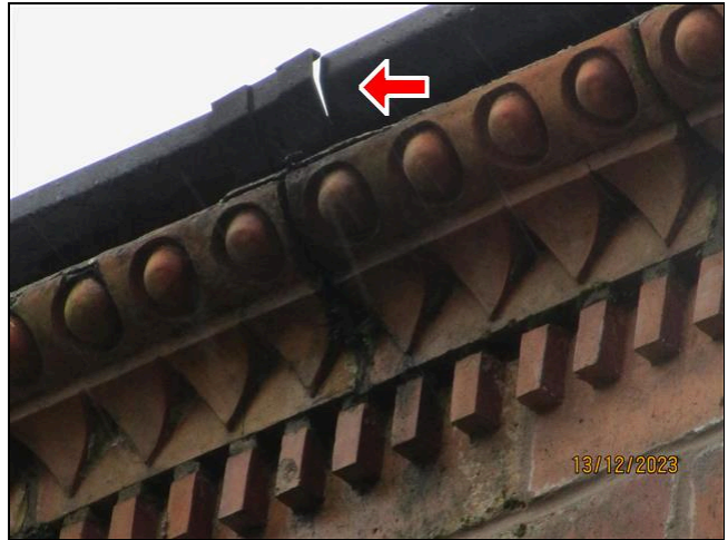
3.0 Item 2(Picture) Gutter leak at the rear
