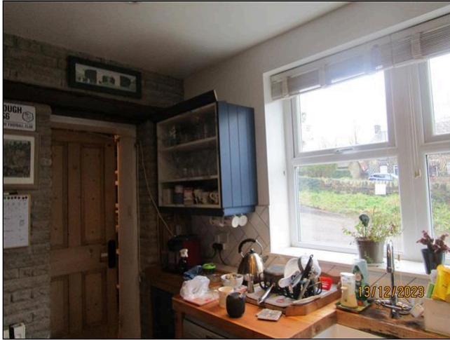
8.2 Item 1(Picture) Windows have no trickle vents
