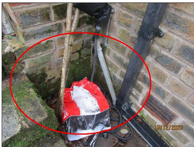
7.2 Item 1(Picture) Penetrating damp to Utility wall
