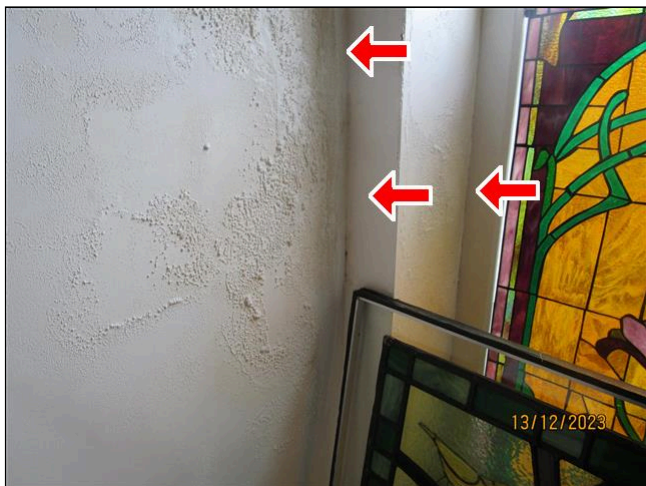
9.2 Item 1(Picture) Damaged wall plaster
